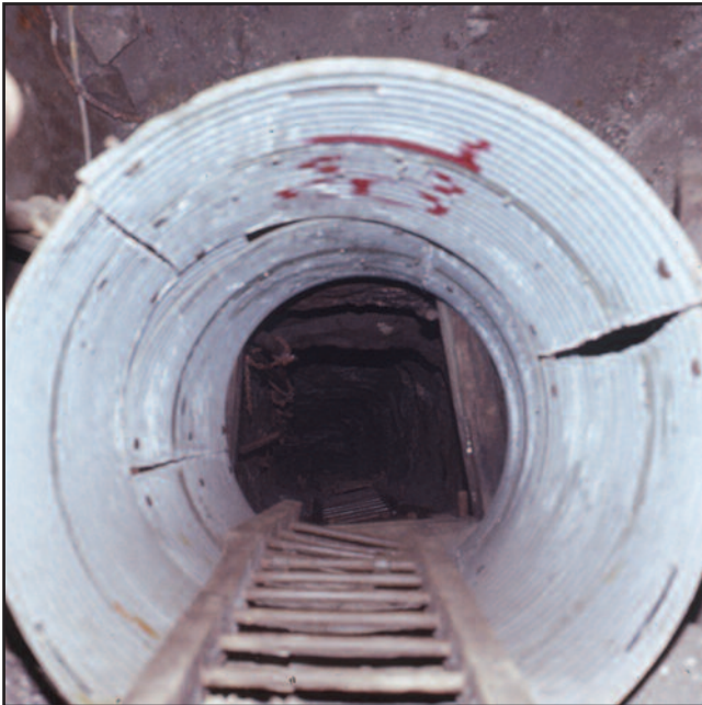
This is a 36-inch corrugated steel ladder-way pipe. There were thousands of feet of these pipes throughout the mine. Every time a mining cycle was completed we would add about 10 feet of this pipe to an existing pipe to advance the ladderway.
