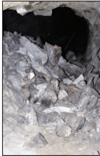
This is what a cave in might look like if we did not scale down or remove the loose rock after a blast.
